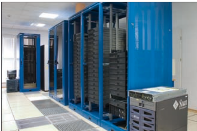
SZB SE cabinets in the server room of the Wrocław University of Technology
