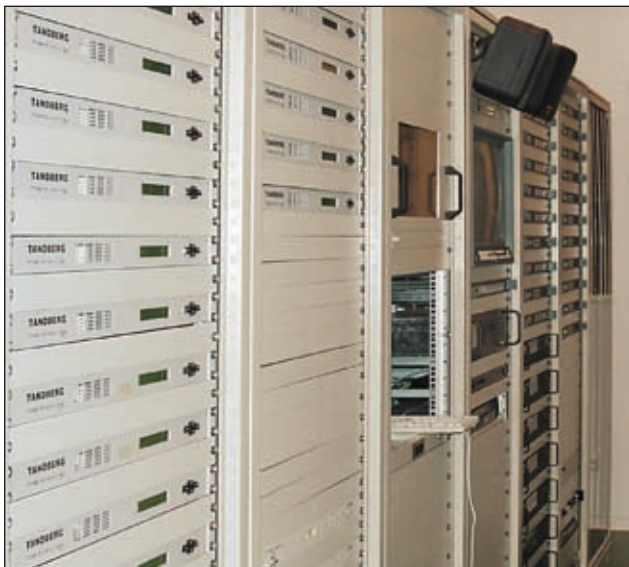
Stub-end station in the branch of Telefonía Polska - Zachód Sp. z o.o. in Stargard Szczeciński. Installation designed and manufactured using SZB cabinets, performed by VECTOR Sp. z o.o. from Gdynia (Poland) - http://www.vector.com.pl
