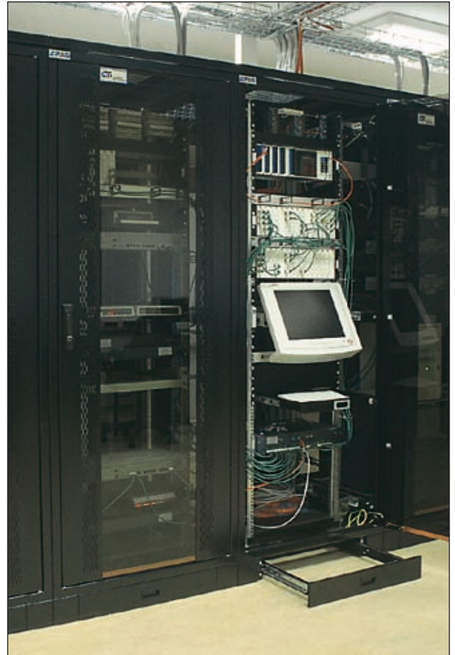
Server room equipped with SZB SE cabinets. Installation was performed by MCP Ltd. from Kraków, Poland ( http://www.mcp.pl )
