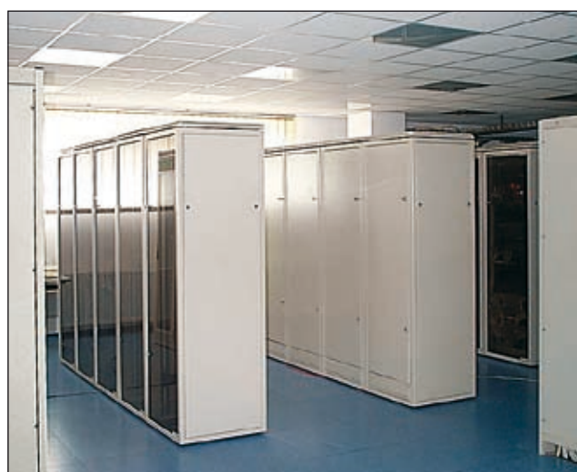
SZB cabinets installed in the headquarters of BPT "TELBANK" S.A. in Warsaw (Poland)
