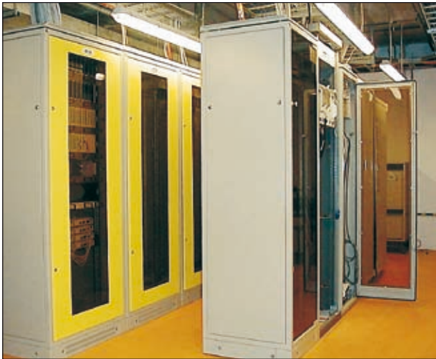
Main distribution room in the Stock Exchange Warsaw building. The whole system is designed and manufactured on the basis of SZB cabinets. Installation performed by ALMA S.A. from Poznań (Poland) - http://www.alma.biz.pl
