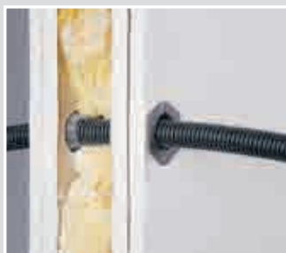
Wall feed-through in plaster-board fire-protection wall.
