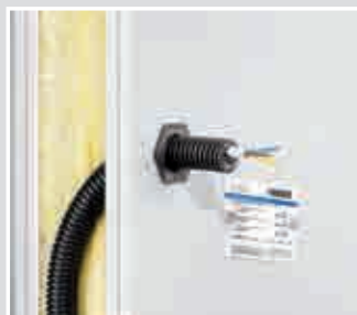
Wall entry with M16-M25 combination entry, in plaster-board fire-protection wall with M25 conduit.
