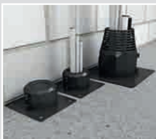
Mixed population of sheathed cables and conduits.
