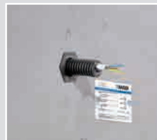
Wall feed-through in concrete fire-protection wall.
