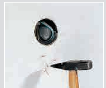
Fine marker bristles on the signal cover show the exact position of the one-gang box after plastering.
