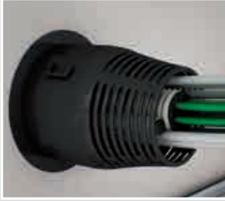
Mixed population of sheathed cables and conduits.
