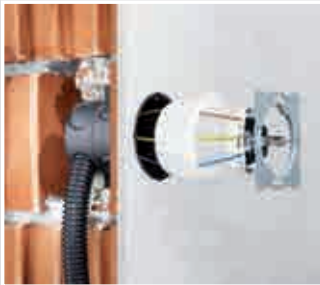
Later air-tight closing of flush-mounting boxes.
