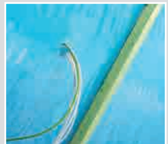
The cables are fed through the building's air-tight seal. This entry must be permanently sealed air-tight.
