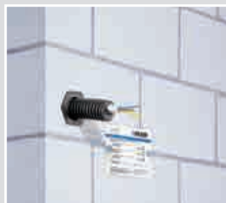
Wall feed-through in sand-lime brick fire-protection wall.
