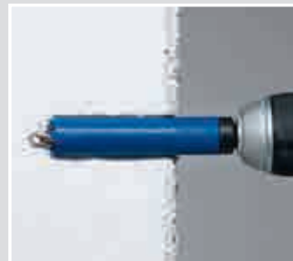
The depth stop ensures that only the amount of insulation needed to secure the mini equipment carrier is removed.
