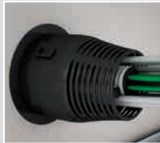
Mixing of cables and conduits.
