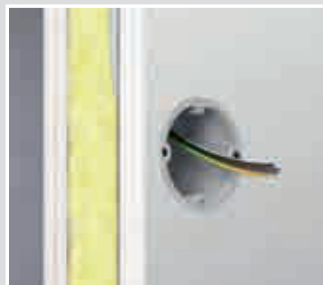
Using the radiation protection box in the wall.
