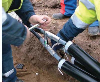
Bolts are tightened using a wrench. It is also possible to use a battery operated wrench.
