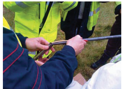
The earthing wire locks in the hardened steel tip with the leading rod.
