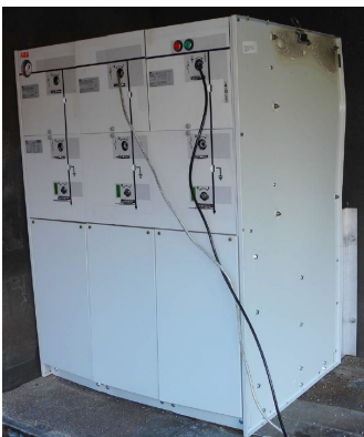
From IAC-test without arc suppressor 20kA/1s
