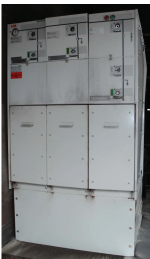
From IAC-test without arc suppressor
